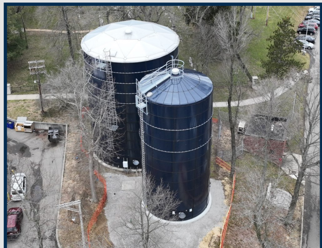
New Water Storage Tank
